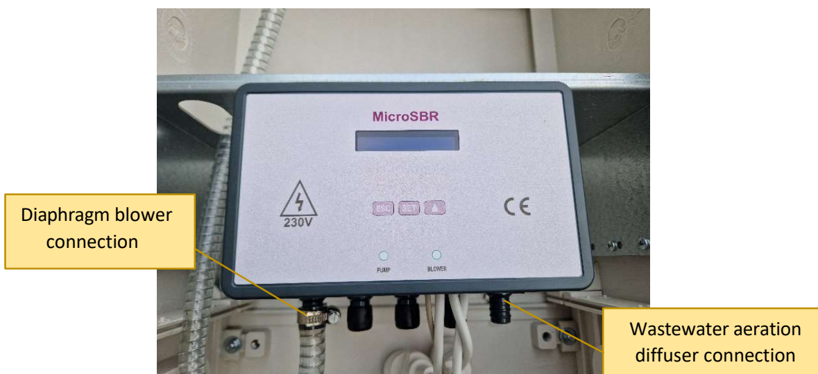
Figure 13: MicroSBR controller of the OPTIMAX VIRO treatment plant
